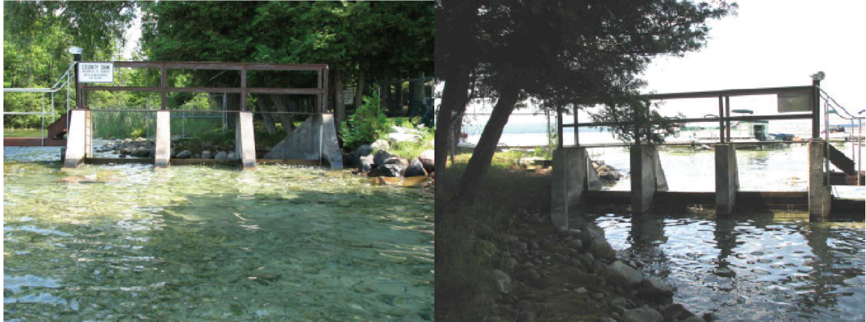
Figure 1.2.2. Image of upstream and downstream side of the stop-log gates (2010 Spicer report). The flow through this section is governed by the use of 5 foot wide wood planks, which are rarely removed due to their unwieldy size and weight.
